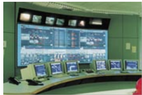
The control room of a waste bunker. If the ThermoVision™ A40 detects a hot spot an alarm will go off.
